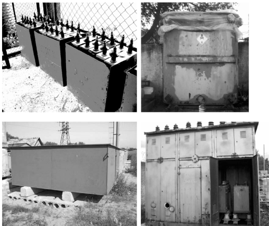
Figure 4. Types of containers for PCB-containing capacitors storage
